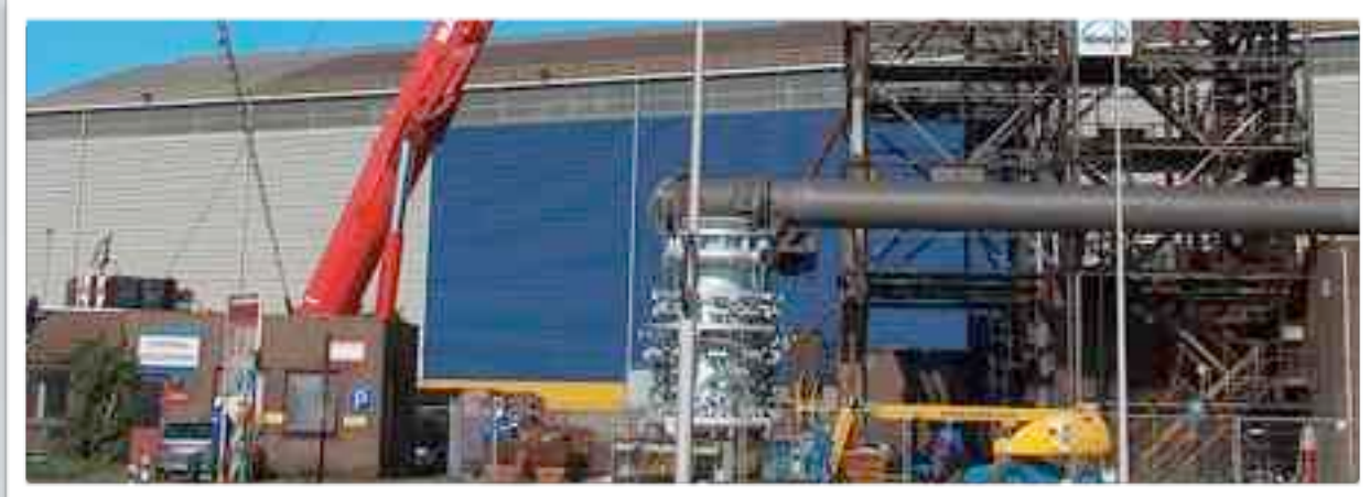
HISarna Blast Furnace (Tata Steel)
